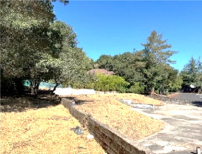
Area 2: Warehouse wall and concrete pad, with rock outcropping to the left
