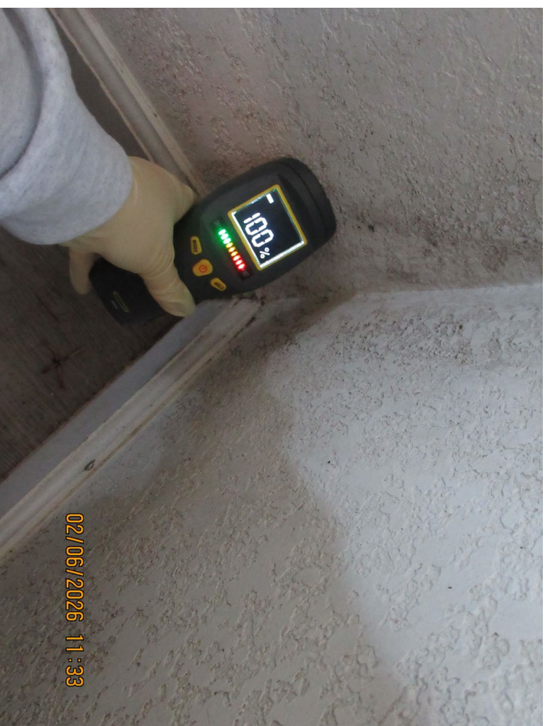
Moisture reading on bedroom wall
