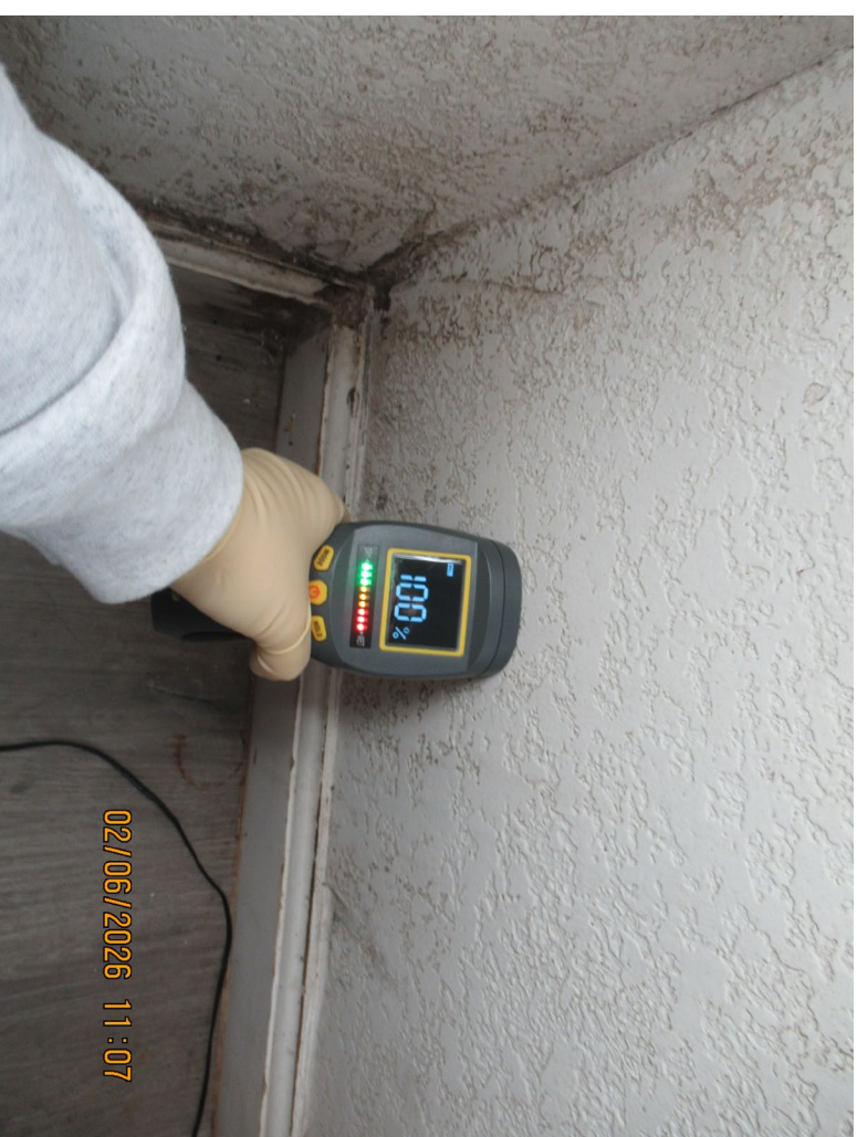
Moisture reading from wall
