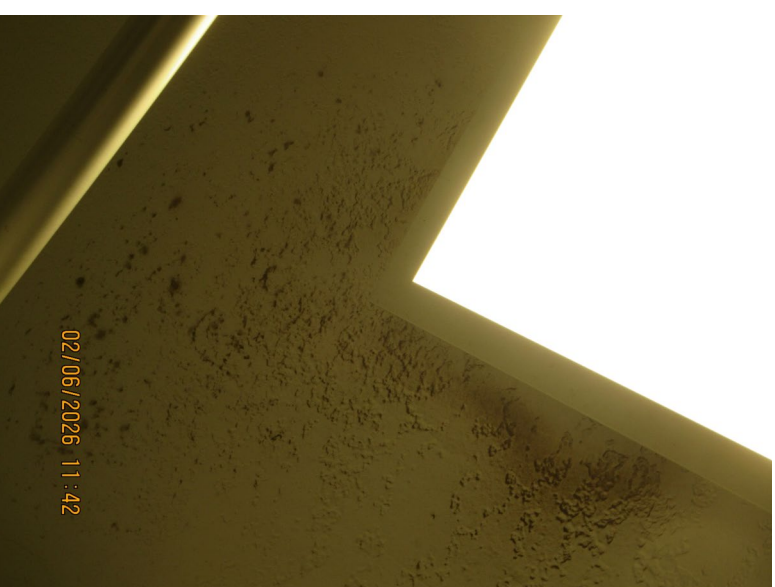
Bathroom light and fan shows buildup on the ceiling
