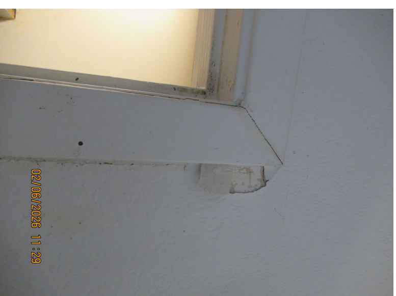
Wall texture peeling around the bedroom door
