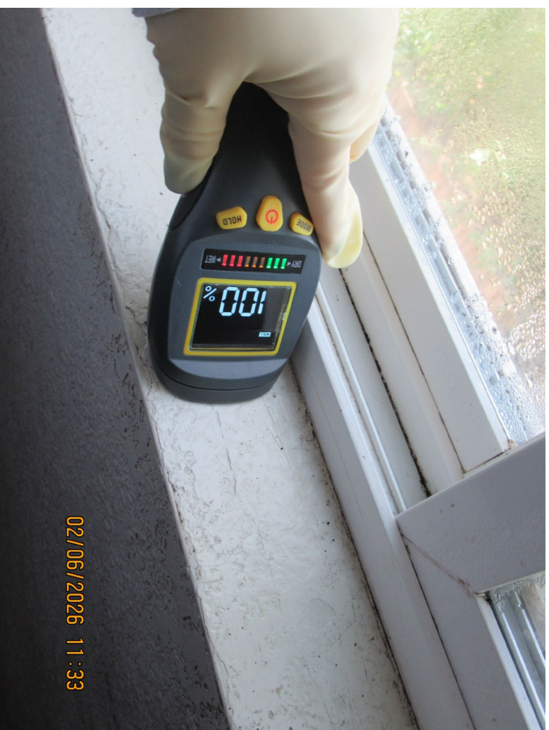
Moisture reading on windowsill
