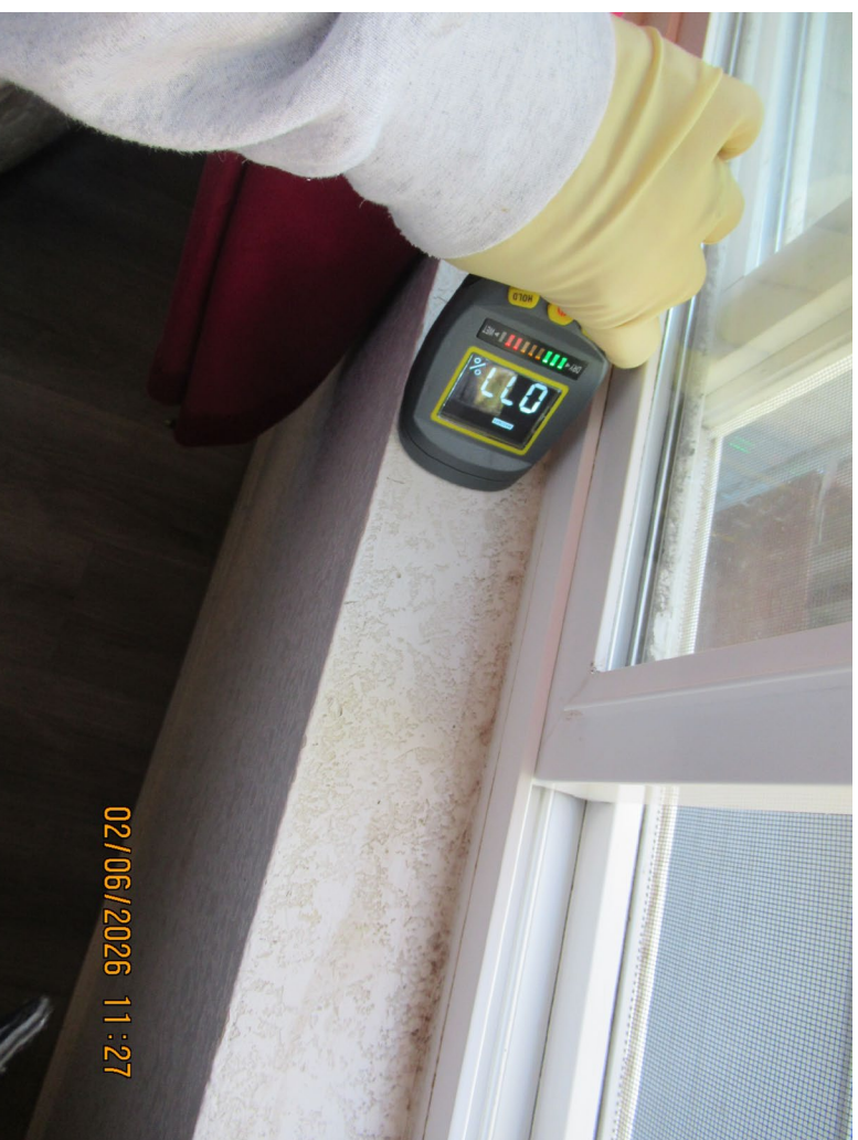
Moisture reading on windowsill
