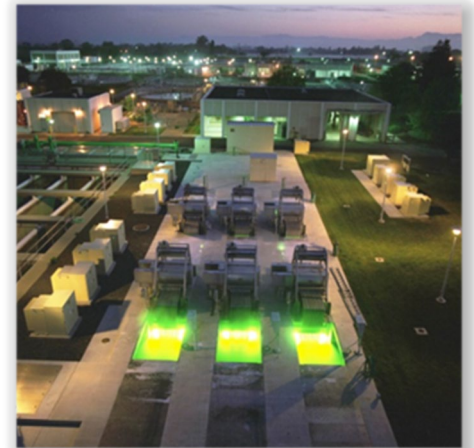
Laguna Treatment Plant
