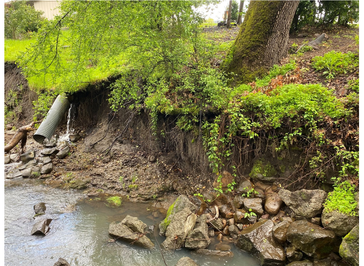
Storm Drain Failure on Oakmont Creek near Meadow Creek Court
