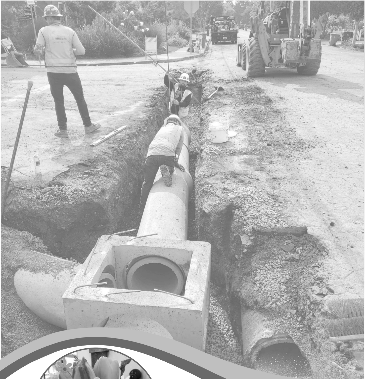
La Paloma, E Havens Water & Sewer City of Santa Rosa
