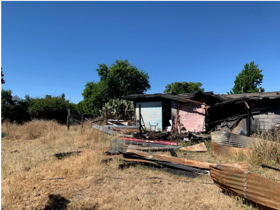
Looking west at the recently burned building and the eastern edge of the project site.
