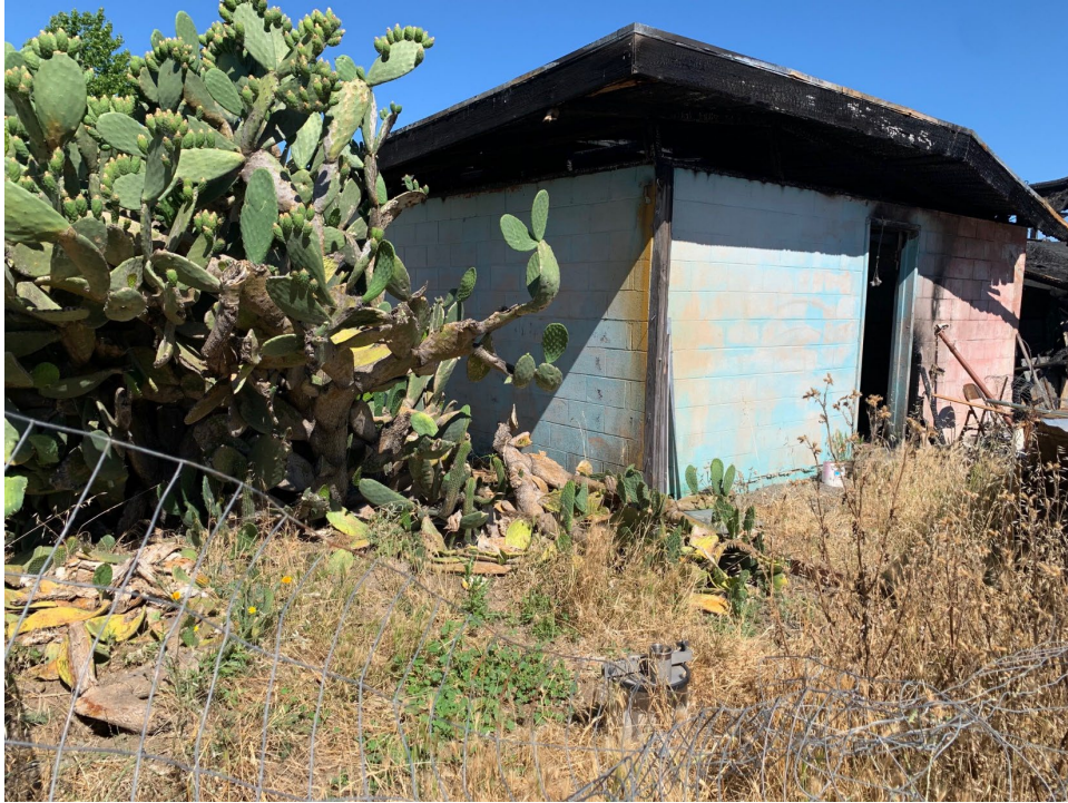
Septic tank area (may be removed) at the eastern edge of the project site.
