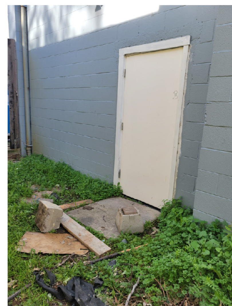
EXISTING CONDITION OF GYM EXITS
