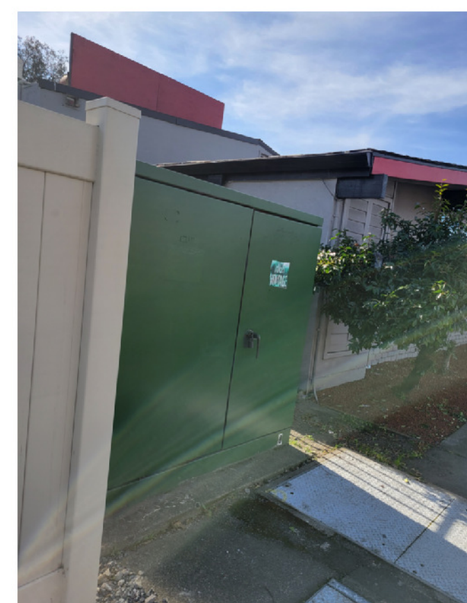
EXISTING POWER BOX BETWEEN SITE AND RESTAURANT
