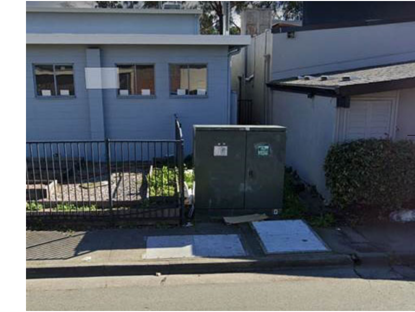
3. EXISTING PGE TRANSFORMER
